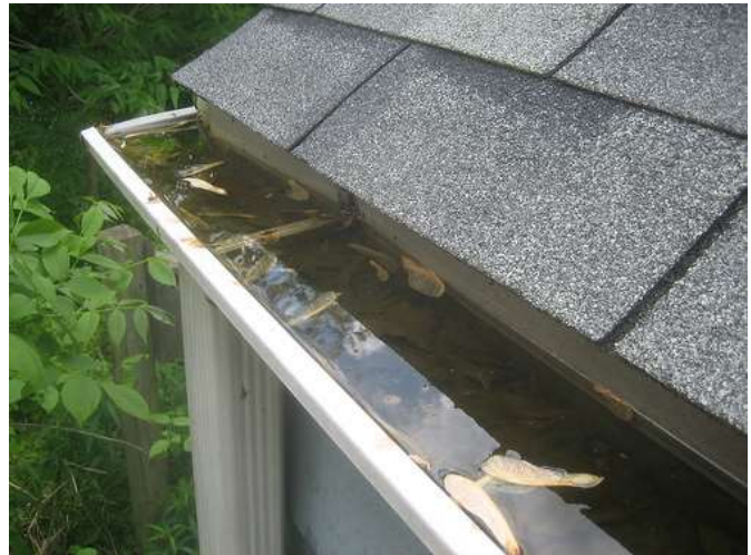
Figure 8. Clogged rain gutter filled with water
