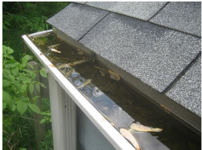
Figure 8. Clogged rain gutter filled with water
