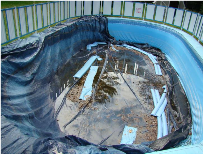
Figure 9. Abandoned swimming pool.
